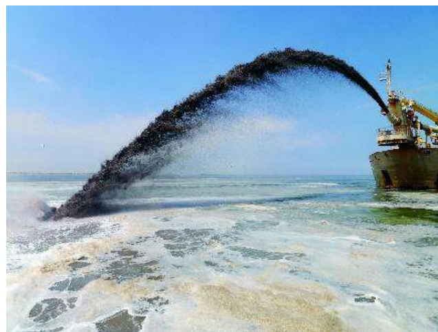
Figure 2-3: Typical methodology for spreading dredged materials at sea. Source: Dutch Department of Waterways and Public Works.
